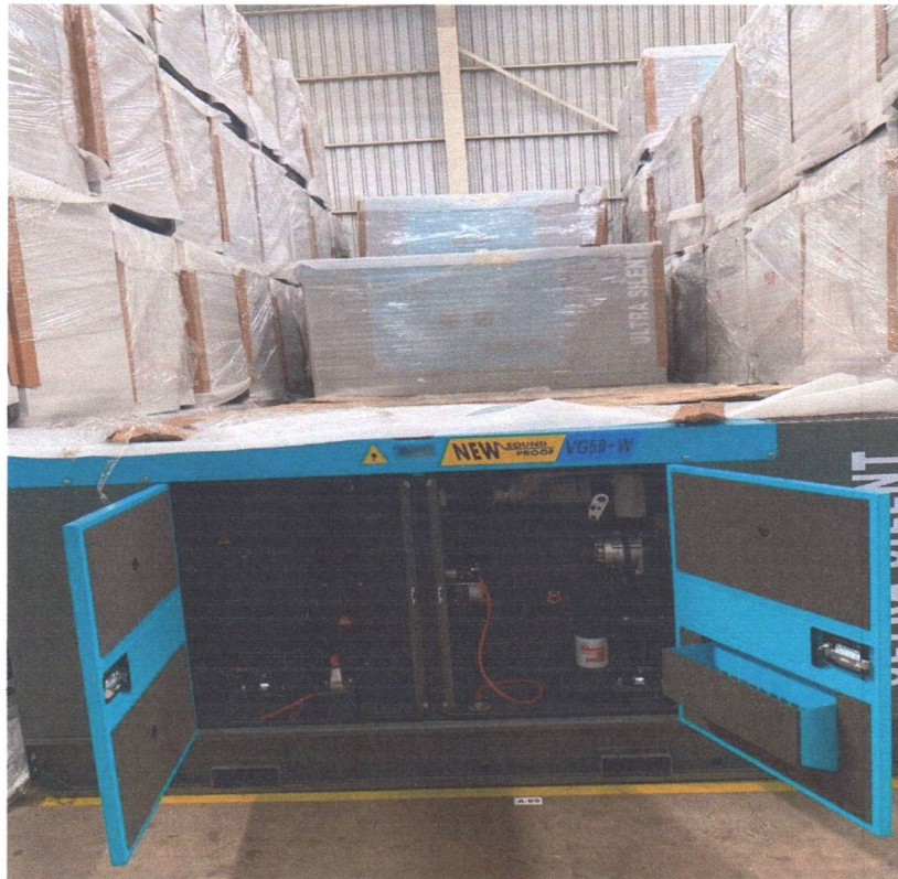
Unit Generator Set
