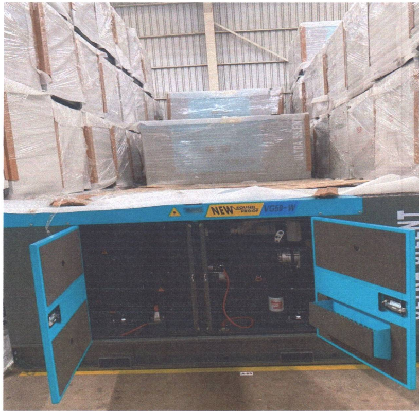
Unit Generator Set
